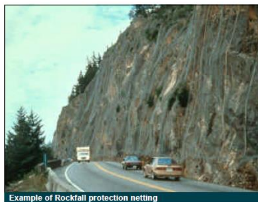
Example of Rockfall protection netting
