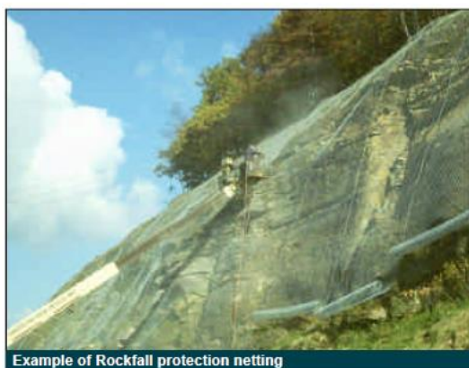
Example of Rockfall protection netting
